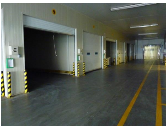
Figure 19 Cold store facility adjacent to a packing house
