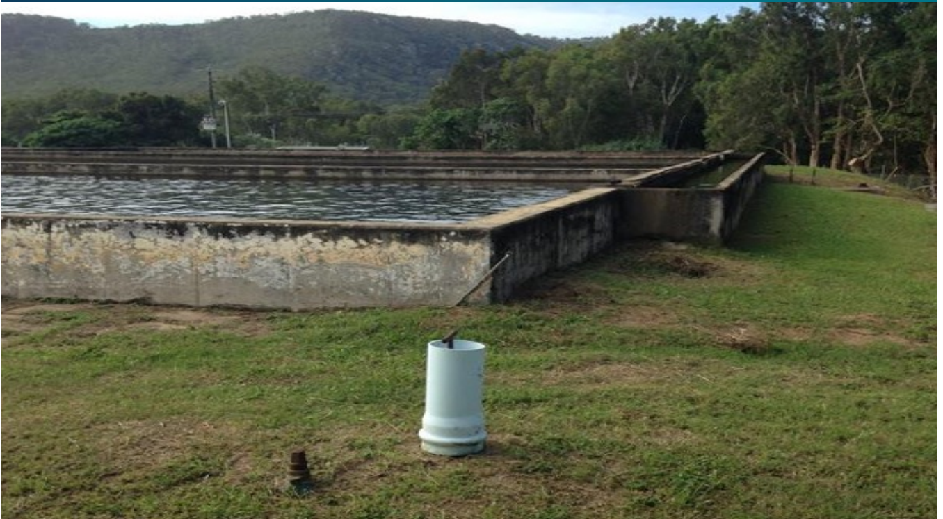
Image: Palm Island Water Treatment Plant. Source: GanDen, n.d.
