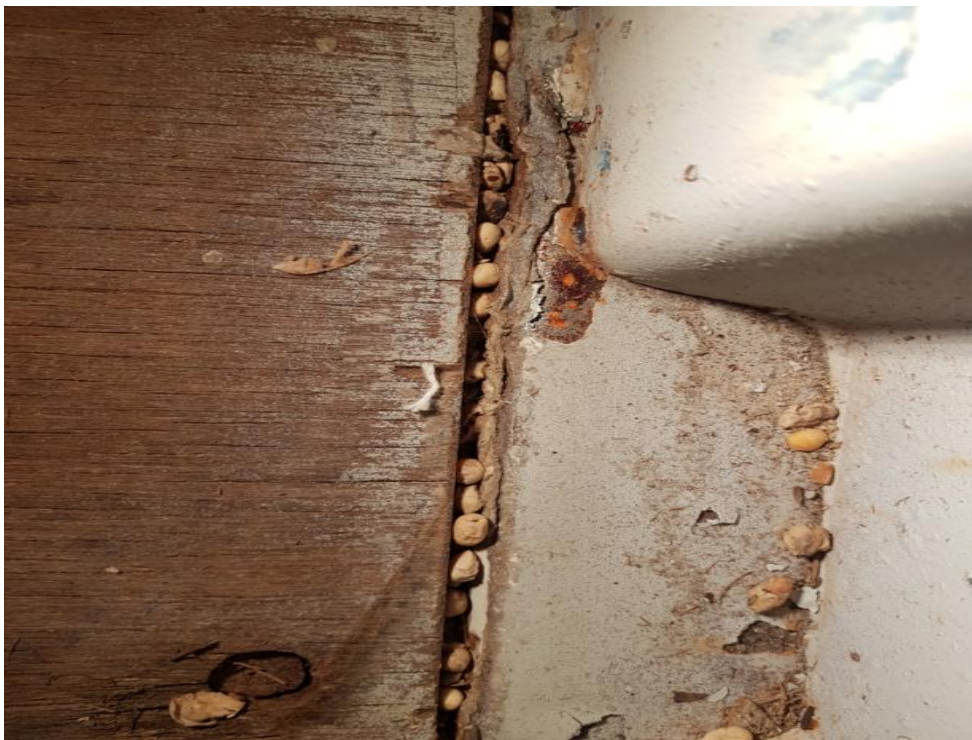
Seeds in interfaces between container wall and floor.
