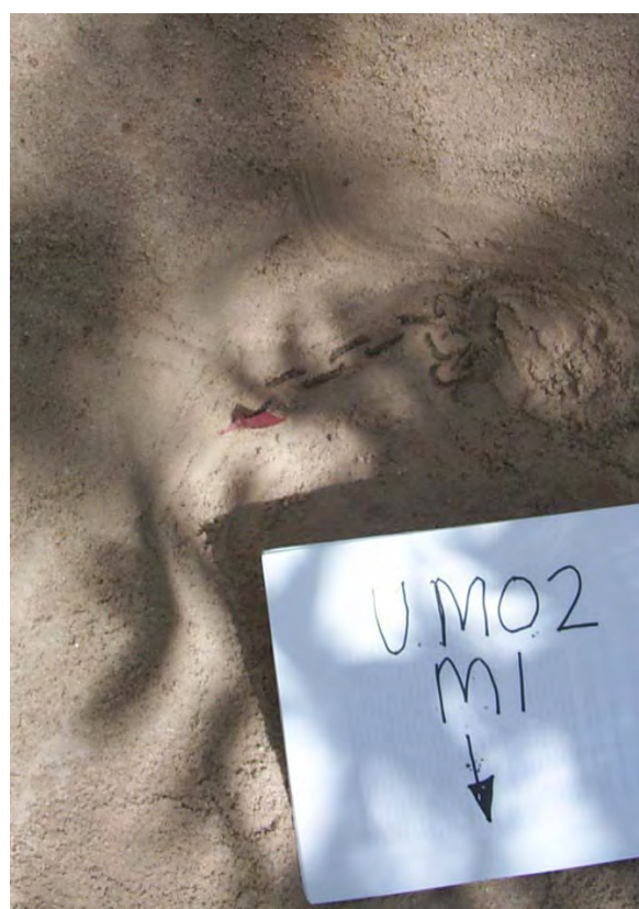
Figure 18 Scour chain UM02-1 (2000) pointing towards the left bank. The flagging tape is attached to the top link.
