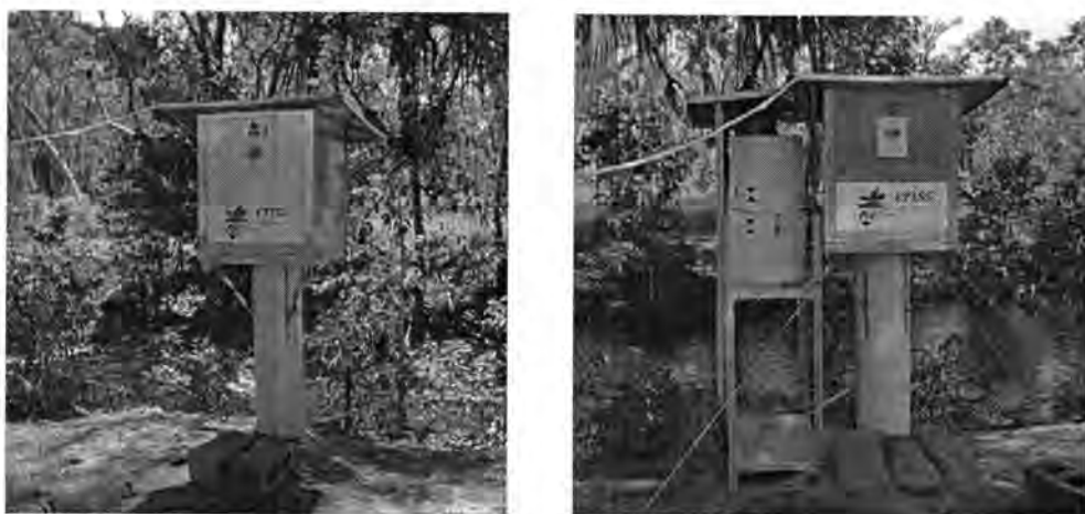
Figure 3 The original completed gauging station (left) and with the additional stand for the second Gamet sampler (right), at Swift Creek
