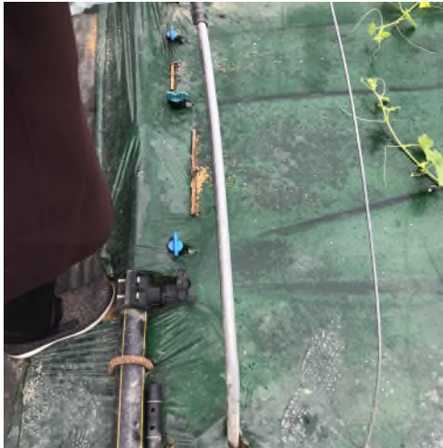
Figure 2.6 Underground drip irrigation system in the greenhouse
