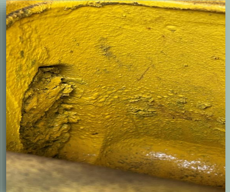
Painted over soil contamination – no attempt to clean
