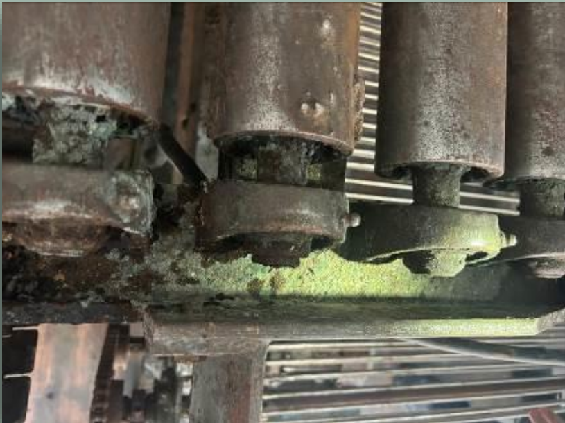
Flour residue and extensive mould on rollers – no cleaning attempted
