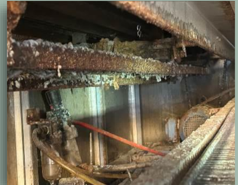
Excessive mould and flour contamination – no cleaning attempted
