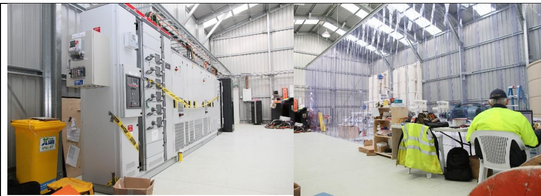
Panoramic of Onshore Plant During Testing
