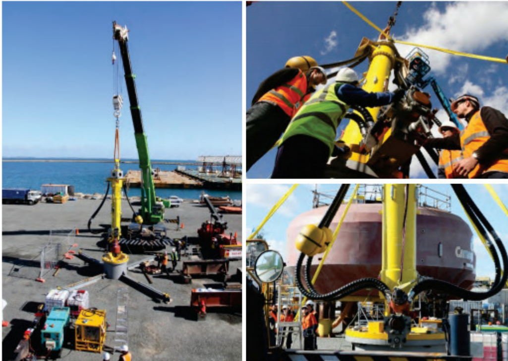
Onshore integration testing of the Pump, Hoses and Foundation Connector
