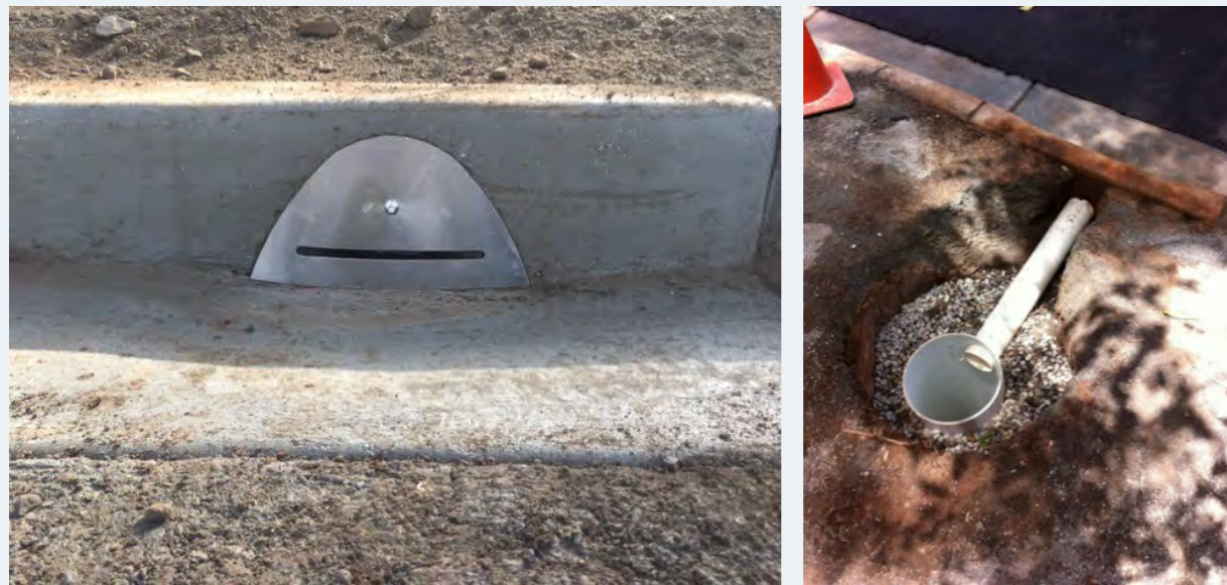
Above images: A TREENET Inlet (pictured above) designed by Space Down Under delivers water to the soil of the street verge (nature strip), providing added water supply for street trees (Johnson, 2022)
