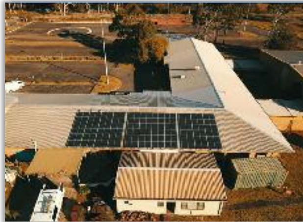
Solar Panels at No.4 Shaft
