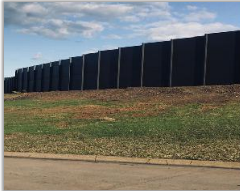
Photo showing recently constructed noise wall at Russell Vale Colliery
