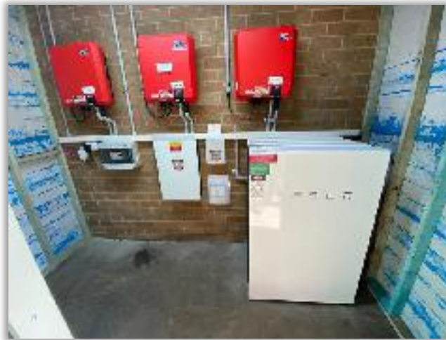
TESLA Batteries Installation
