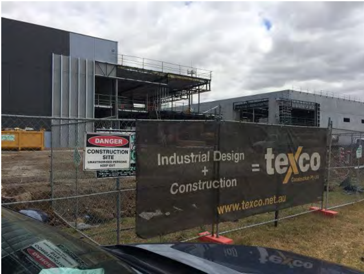
All NTGVVP has been removed from the site. Construction of warehouses is underway
