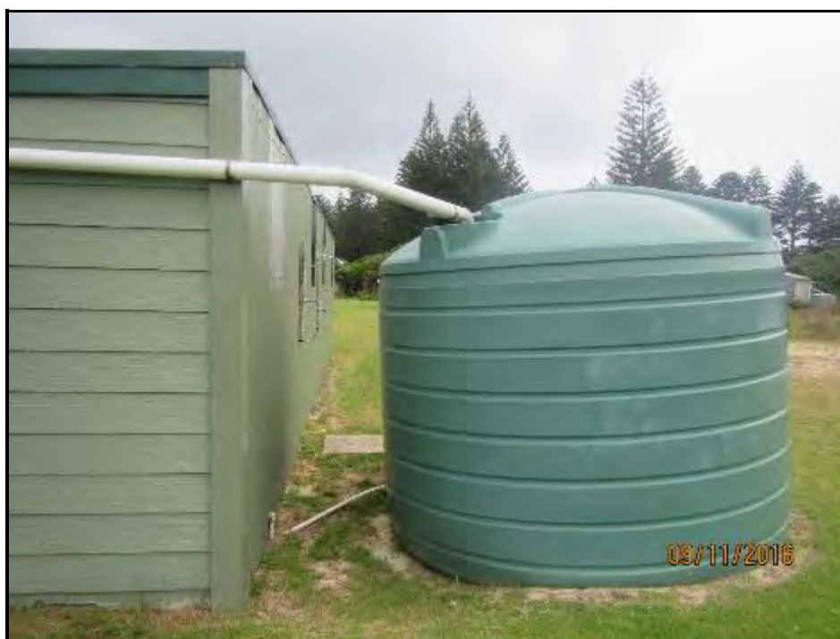
Photo 22: Example of a rainwater tank collecting water from a roof surface
