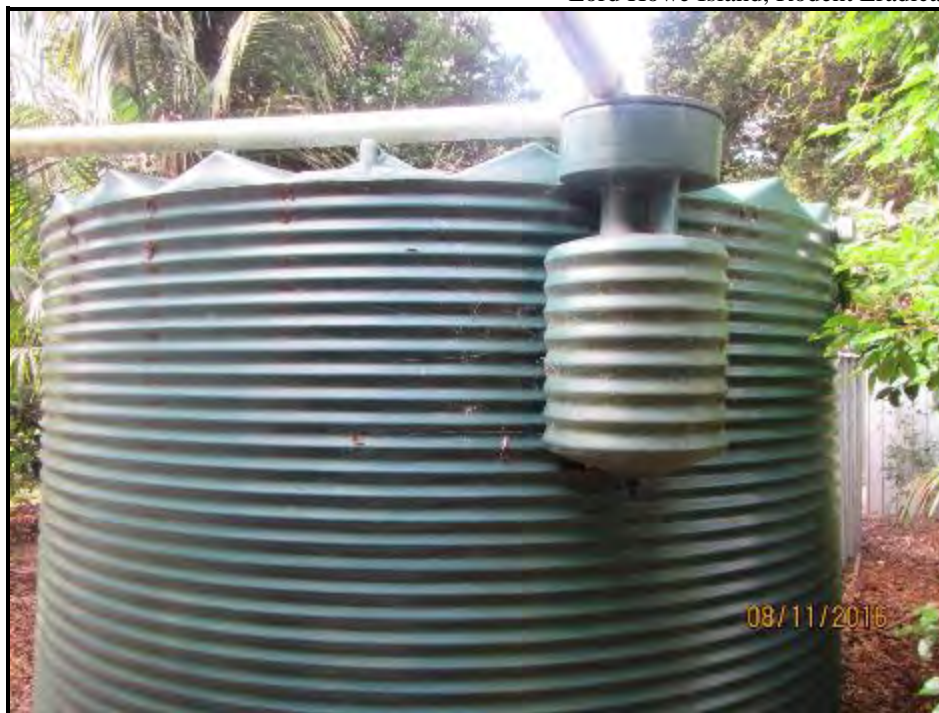
Photo 21: Example of a rainwater tank with first flush/sedimentation tank
