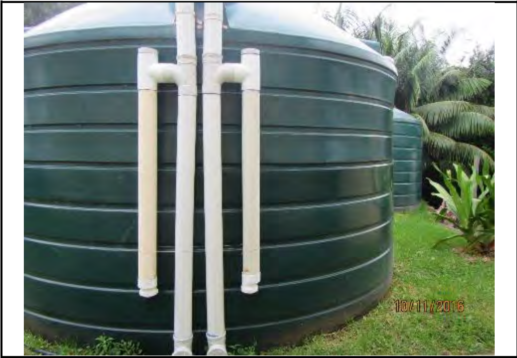
Photo 19: Rainwater tank with 'first flush' system
