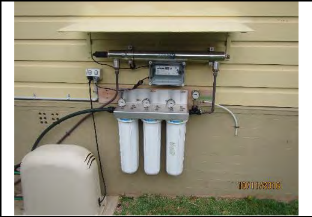
Photo 20: Groundwater filtration unit owned and operated by LHIB
