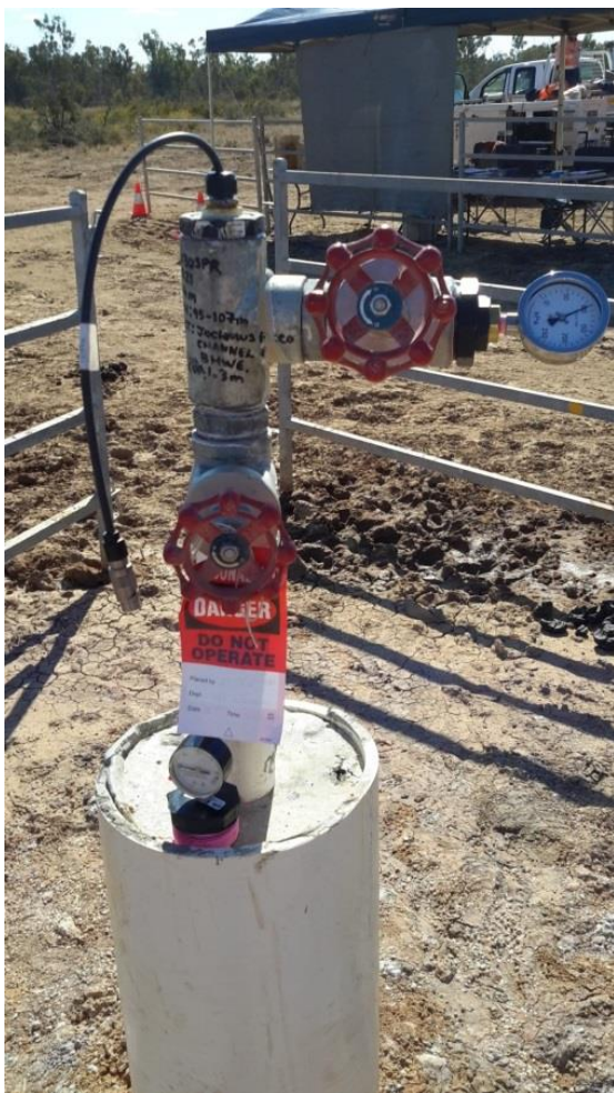
Figure 21 Artesian Monitoring Bore Headworks
