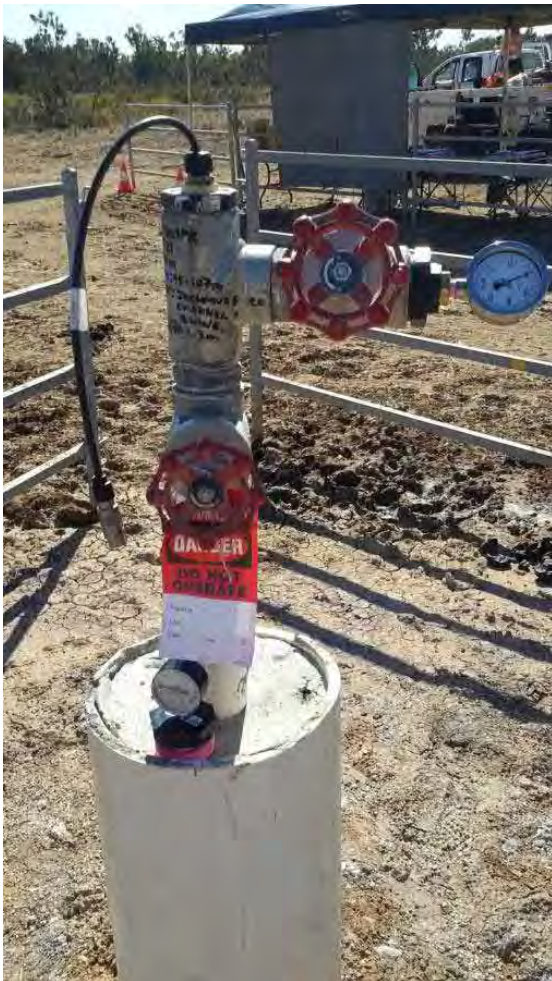
Figure 21 Artesian Monitoring Bore Headworks
