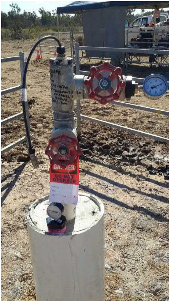
Figure 21 Artesian Monitoring Bore Headworks
