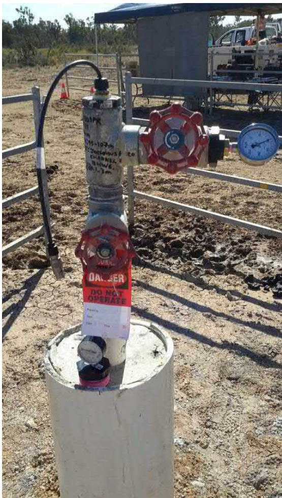
Figure 21 Artesian Monitoring Bore Headworks
