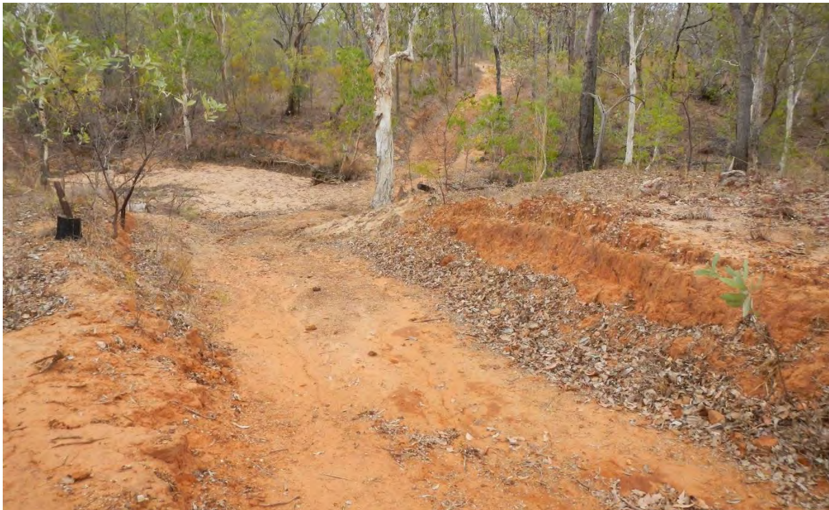
Figure 14 A road cut through a creek crossing near Area 1 that is accelerating rill and gully erosion.
