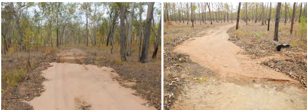
Figure 12 Sand/silt infilling a ‘whoa boy’ in Area 1 from excess water runoff and infrequent whoa boy placement.
