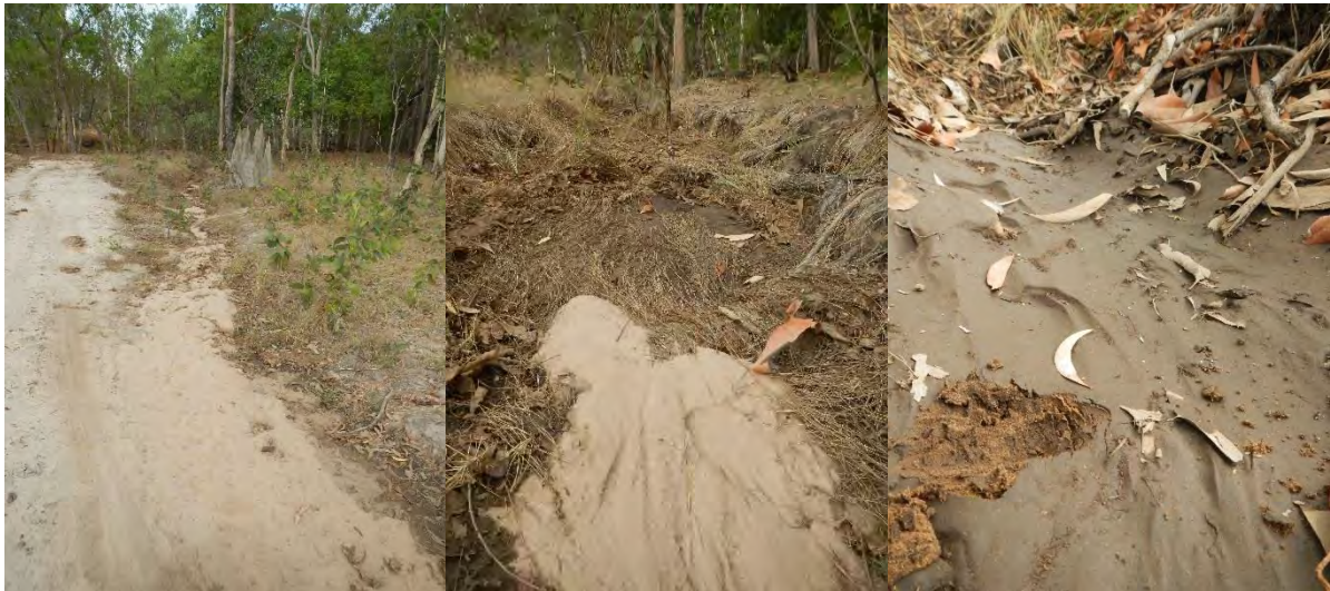
Figure 13 A cut drain off a track in Area 1 delivering sand, silt and clay directly into an adjacent waterway.
