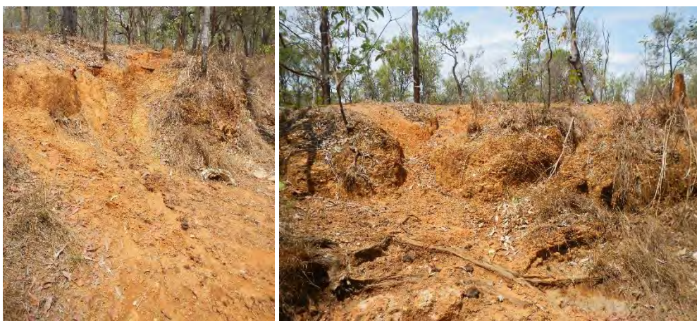
Figure 16 Rill and gully erosion along the banks of Jones Creek enhanced by cattle pads, trampling and local overgrazing.
