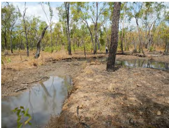
Figure 19 Channel and gully erosion into a dambo valley downstream of a farm dam and road crossing.
