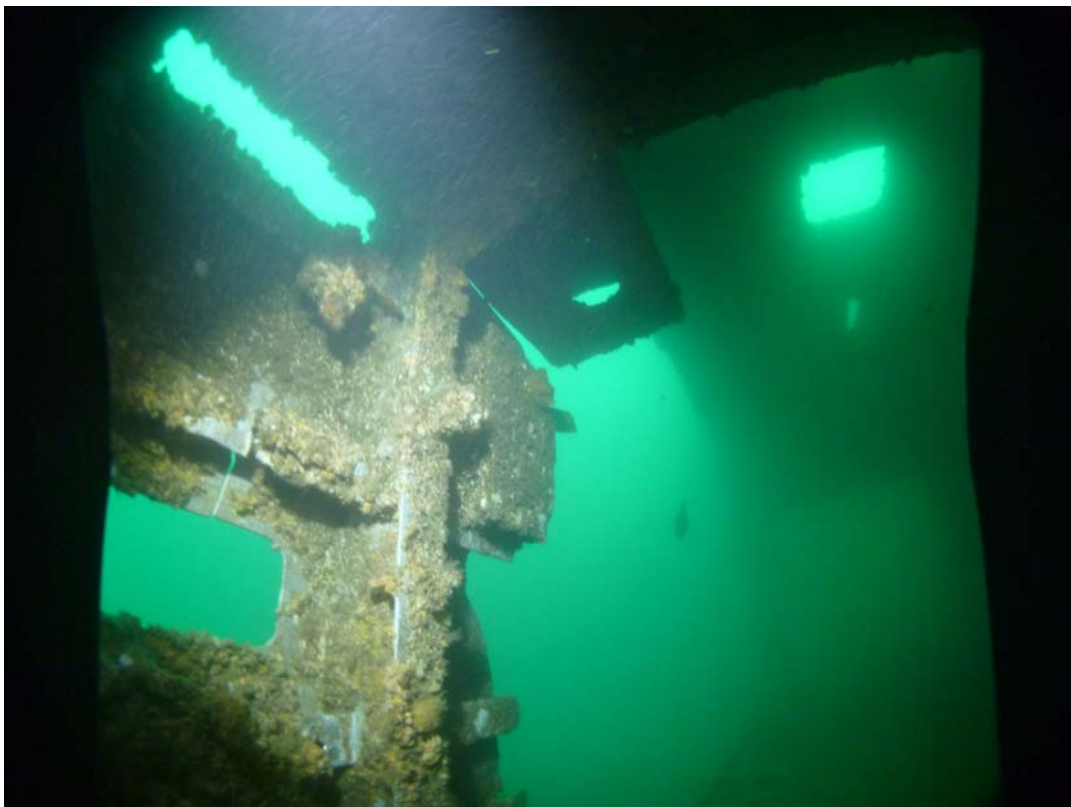
Photo 2: This photo of the EX-HMAS Adelaide is looking aft from inside the starboard hanger, it shows the area of the hanger side whereby the side has parted from the main structure
